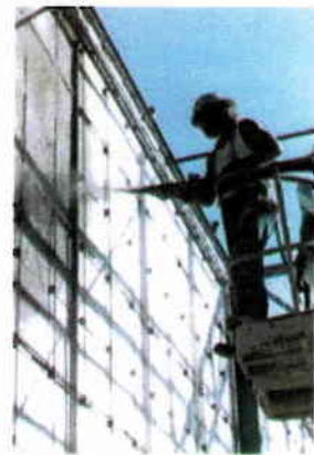
After erecting prefabricated panels at the construction site, contractors create the concrete layers by spraying shotcrete
